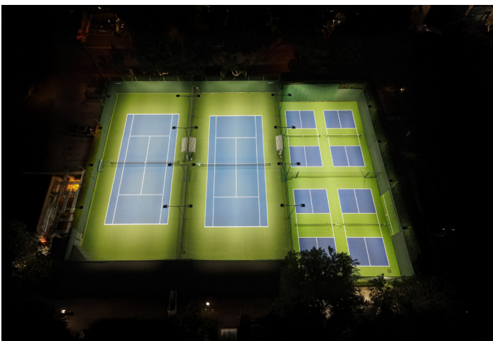
The Valley Hunt Club | Pasadena, CA Installed Lighting System: ProCourt
