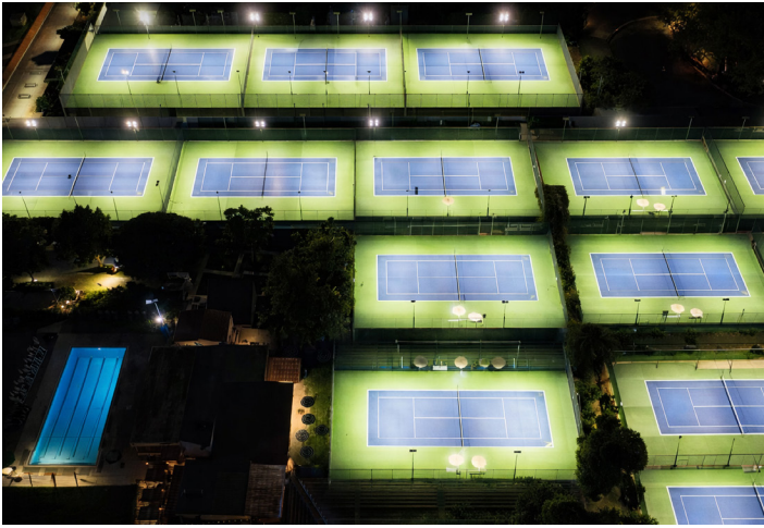
Newport Beach Tennis Club | Newport Beach, CA Installed Lighting System: ProCourt
