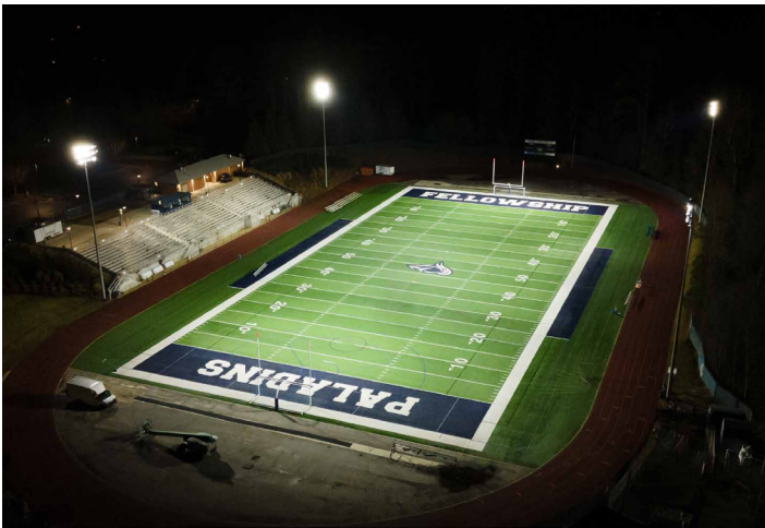
Fellowship Christian School | Roswell, GA Installed Lighting System: Liberty
